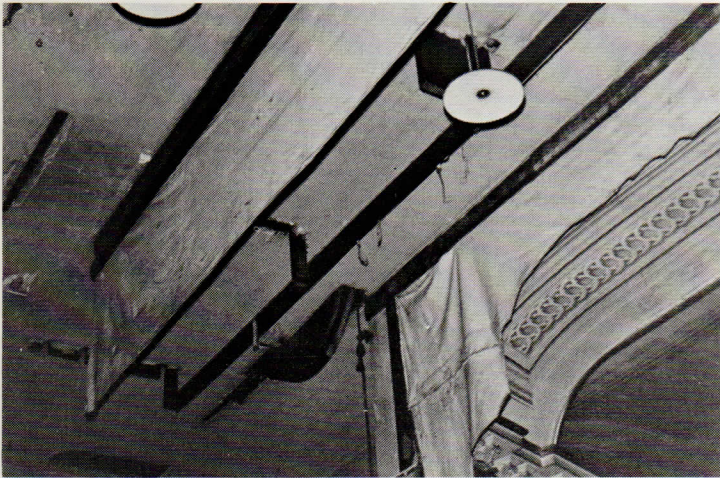
Stage ceiling showing the remains of borders and the pulley used in raising and lowering the grand drape. Electric light fixtures are obviously a late addition.
