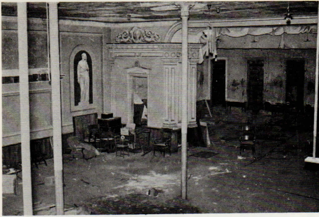
Remains of the auditorium as seen from the level of the balcony. Looking to the stage area, it is evident the raked stage flooring has been torn out as has the balcony itself.
