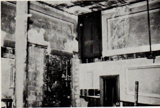
The door opening at ceiling level was the entrance to the balcony. Door at floor level opened into a cuddy in which kerosene footlights were stored. The balcony was suspended from the hanging metal supports shown in both views.
